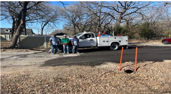
Hunt County Road Crew works on curve at CR 2451 to reinforce the culvert and roadway.
