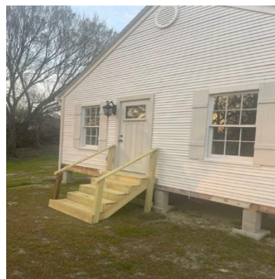
Council member Tom Anderson donated wood and time to build the steps to the back door at the Town Hall!
