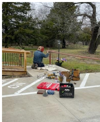
Mike Durrett, an accomplished welder from Wills Point completes the required ADA loop railing at Town Hall.
